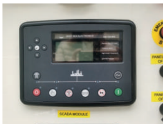
1-EMS control system
