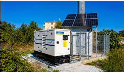
Türk Telekom Mobil İletişim Hizmetleri Country: Türkiye Sector: Telecom Generator: 3 x AC 2700, 2 X APD 25 A, 86 x APD 25 BD Total Power: 8.4 MW
