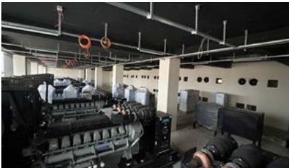
Mardin 750-Bed City Hospital Country: Türkiye Sector: Construction Generator: 6 x AP 2500 Total Power: 12 MW
