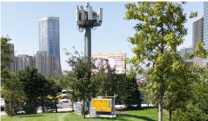
Türkcell İletişim Hizmetleri Country: Türkiye Sector: Telecom Generator: 307 x APD-T 22 BDS3A-M, 170 x APD-T 36 BD-S3A-M, 3 x APD-T 55 BD-S3A Total Power: 10.4 MW
