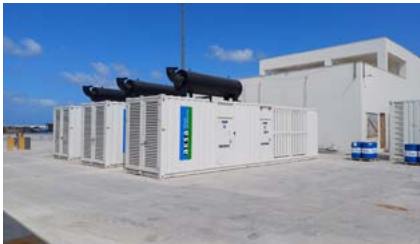
Libya Benghazi Terminal Port Project Country: Libya Sector: Construction Generator: 5 x AP2500, 4 x AP1650 Total Power: 15.2 MW
